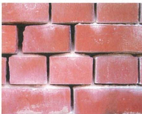
This wall has a severe case of rising damp and salt attack and needs urgent attention. While it may seem that there is a problem with the mortar, in fact the permeable lime mortar has protected the bricks by acting sacrificially. The correct approach to repair is to repoint the joints in a lime mortar. (Photograph David Young)
