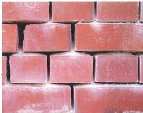
This wall has a severe case of rising damp and salt attack and needs urgent attention. While it may seem that there is a problem with the mortar, in fact the permeable lime mortar has protected the bricks by acting sacrificially. The correct approach to repair is to repoint the joints in a lime mortar. (Photograph David Young)
